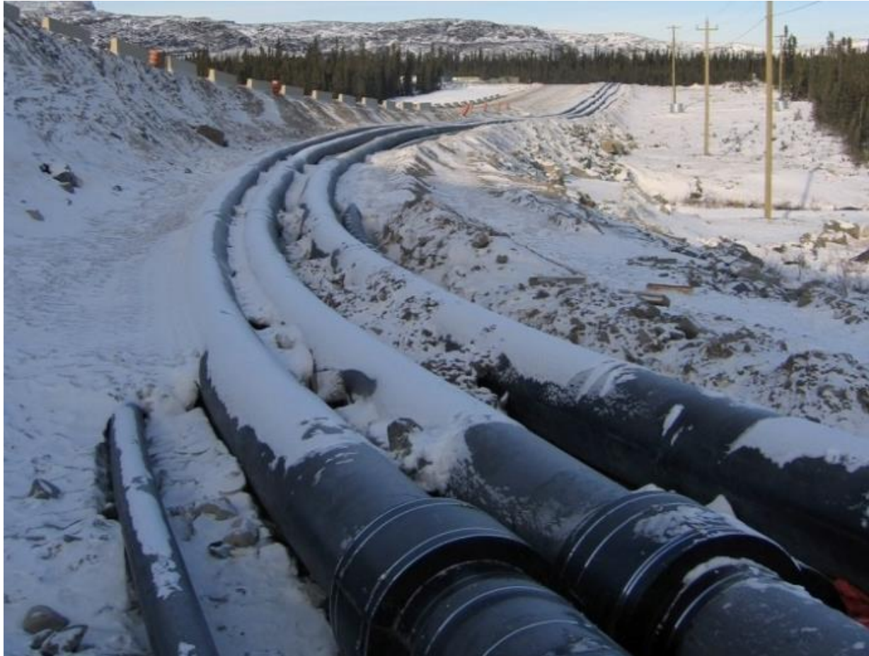
Freeze control pipes
